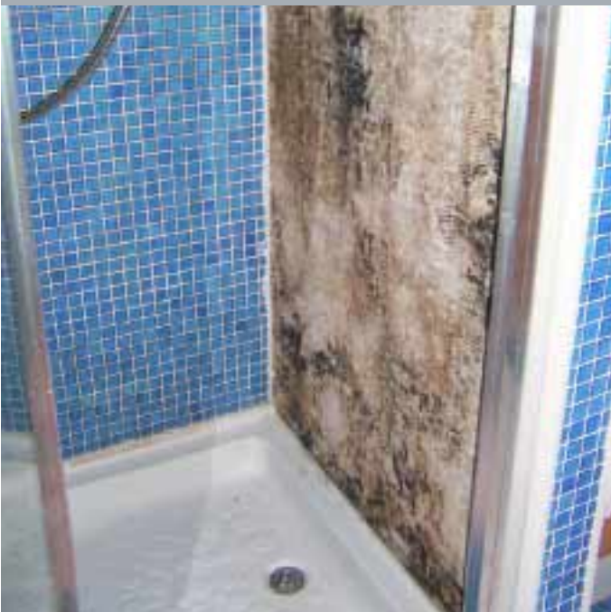
The result of tile failure on a traditional substrate
